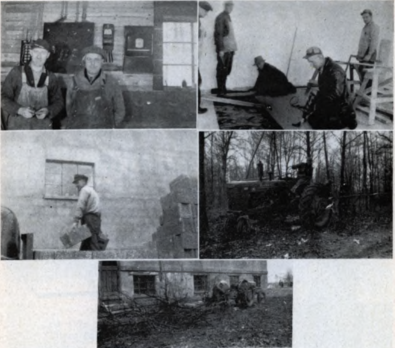
Electricians . . . Laying the hardwood floor . . . John Dick unloading cinderblocks . . . Thinning the bush . . . Cleaning the campus.
