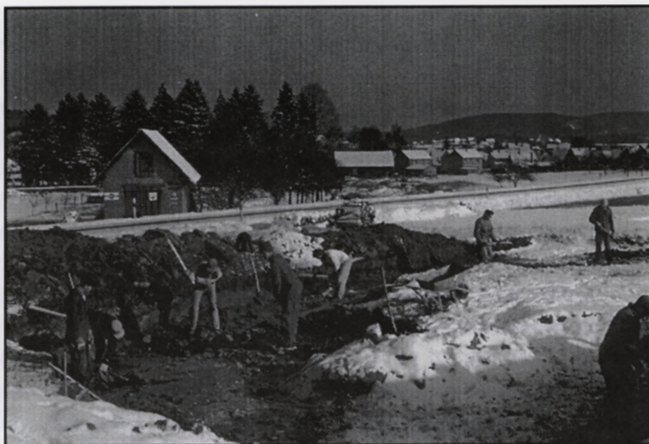
Ernie Toews and others, digging footings in the rocky soil. (Courtesy Ernie Toews)
