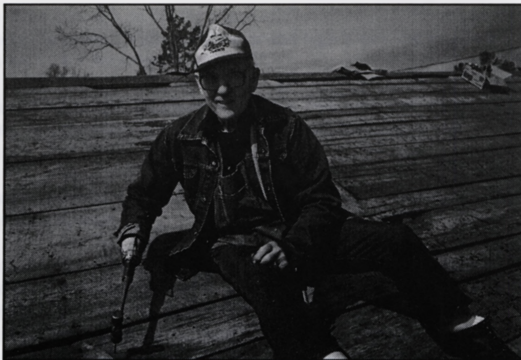
Frank Butterfield from Michigan prepares a roof for new shingles (Courtesy Harry & Louise Block)
